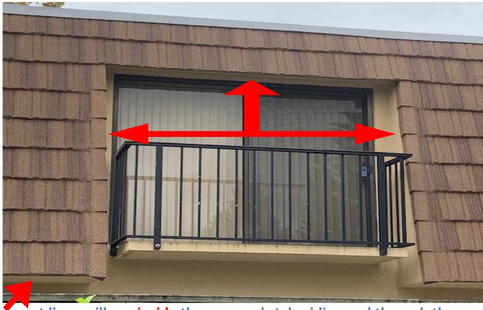
Figure 4 - The refrigerant lines will run inside the mansard style siding and through the overhang in order to be able to connect to the air handler which is located on the second level (as shown with the red arrows) .
